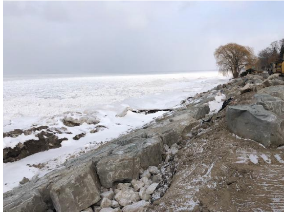
Here, the seawall is starting to take shape just west of Penhuron Drive.
